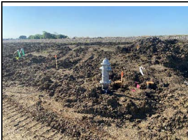
Fire hydrant in subject
