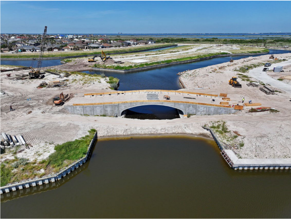
View of Improvement Area #1 between Harrier Point and Whitecap Island facing northwest toward Corpus Christi Bay
