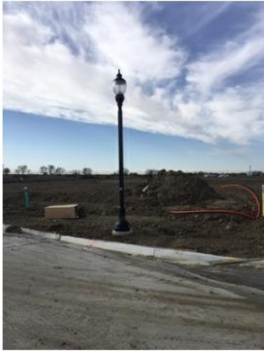
Street Lights Installed In Phase 1
