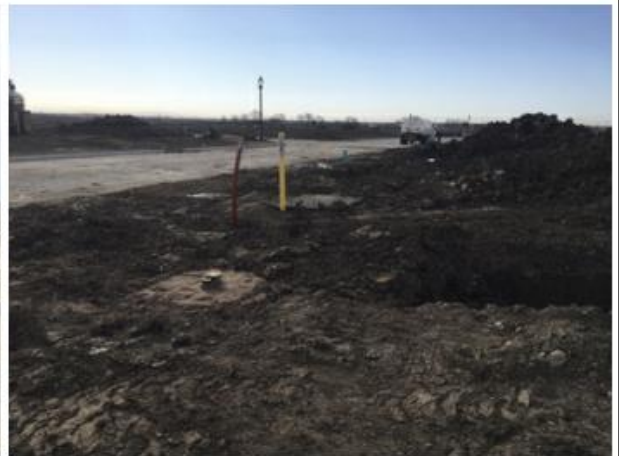
Natural Gas Pipeline Near Main Entrance Off FM 1305
