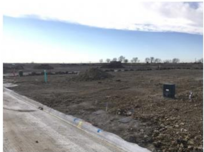
Water, Sanitary Sewer, Electric, Natural Gas, Telecom And Storm Sewer Appear To Be Complete
