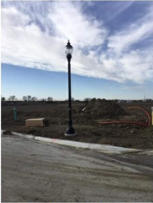
Street Lights Installed In Phase 1
