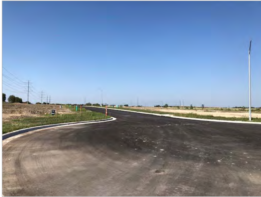
Infrastructure in Place
